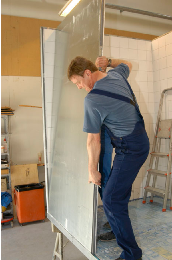
Figure 1. Mounting of a wall element. The elements are mounted in a groove running along the edge of the floor eleme.
