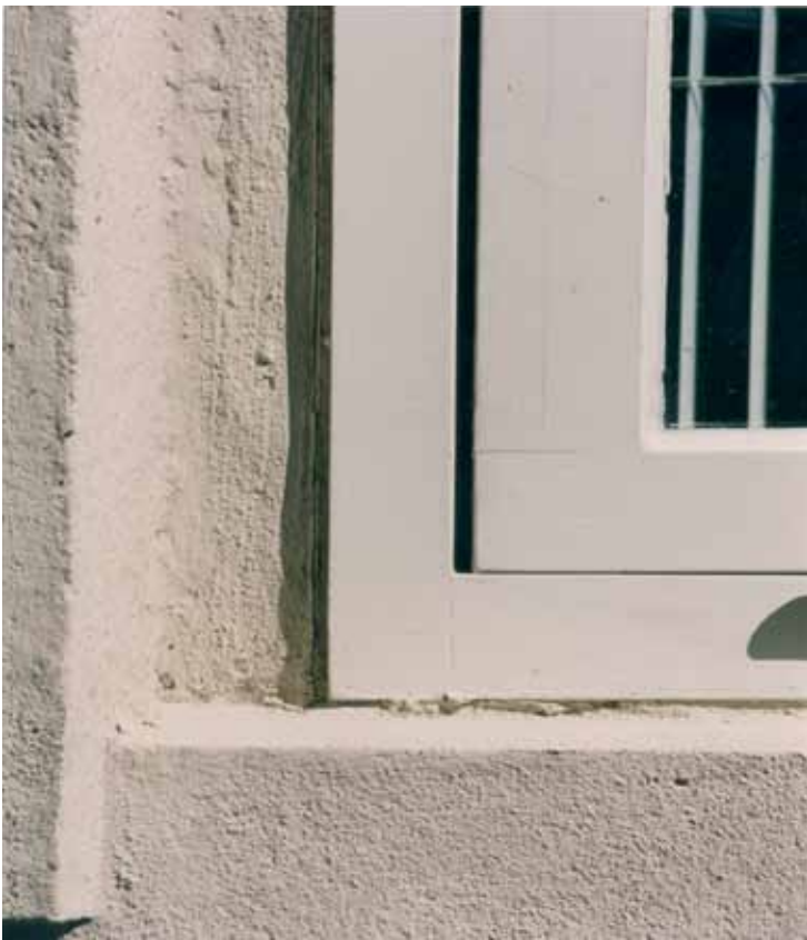
Fuge mangler under vindue
