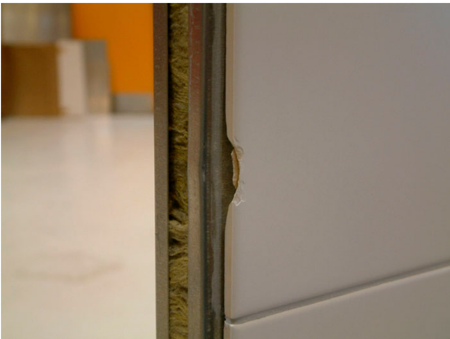
Figure 5. Tile on edge of wall element after impact from steel ball (15 Nm).
